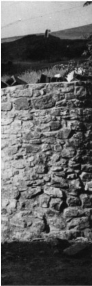
By July, 1970, the Llorente home was well on its way to completion. Above the wall, left center, can be seen the apple tree and beyond that, the pines.
